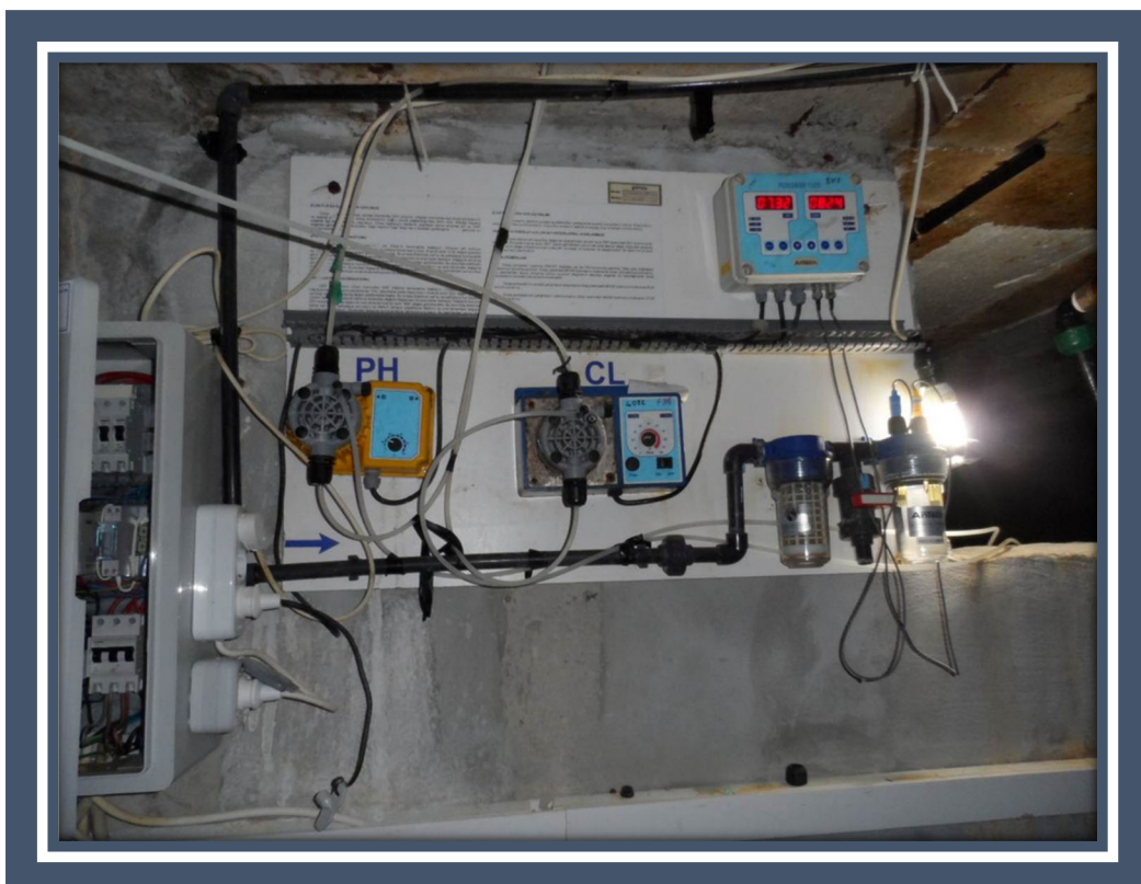
PICTURE: POOL CHEMICAL AUTOMATIC DOSING SYSTEM
